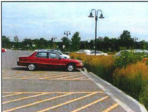
Interlocking concrete pavers with curb inlets to direct rainwater to bioretention area
