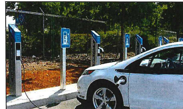
Electric Car Charging Station
