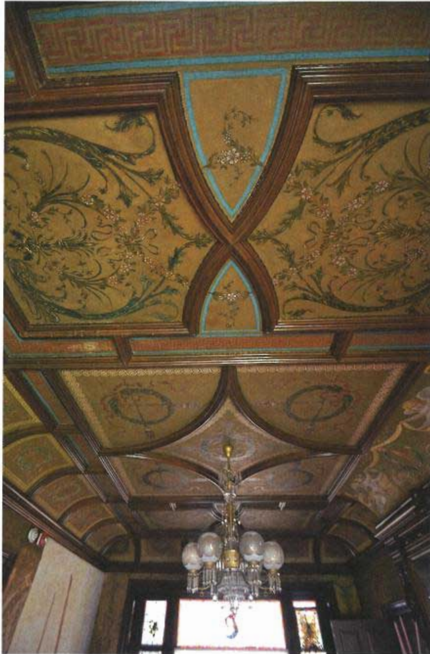
First floor dining room details: Ceiling detail, facing north. Chandelier is not believed to date to the Mattison era and is not a protected element of this easement.
