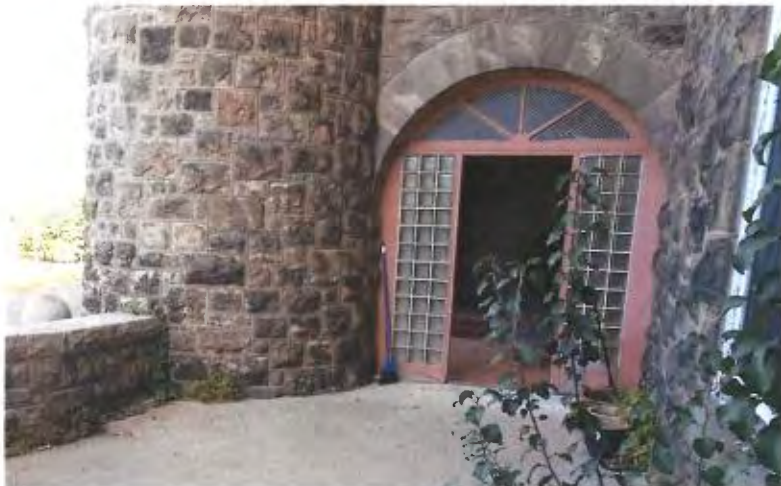
West Elevation Details: An arched doorway connects porch to a raised, open patio to its north. The doorway features a glazed fanlight transom and glass block sidelights in wood frames, but no central leaf. The patio features a concrete floor and a low stone-capped perimeter wall.
