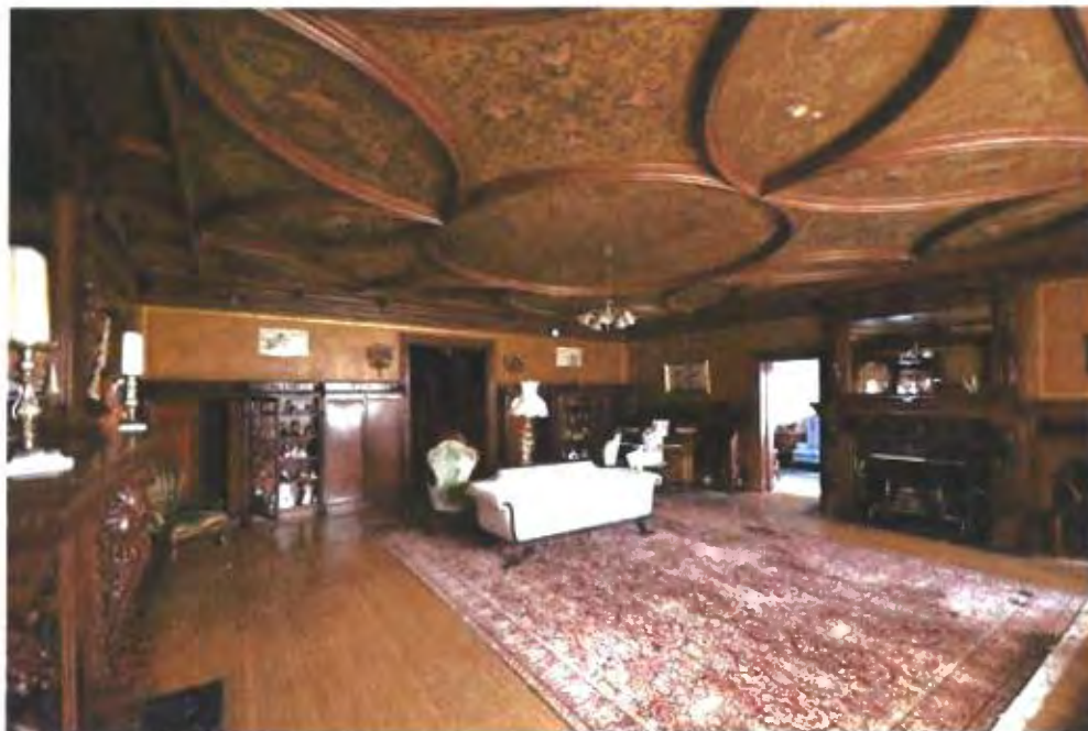
Second floor front parlor: Facing southwest (top); facing southeast (bottom) Light fixtures do not date to the Mattison era and are not protected elements of this easement.
